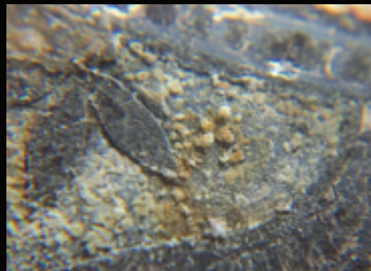
Fig. 1: White deposits leaching from the base metal
